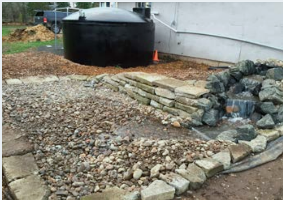
Figure 1. Two rainwater-harvesting systems were built at the Oregon State University's Oak Creek Center for Urban Horticulture. A pond-less waterfall system (foreground) was built next to an aboveground cistern system (background).
