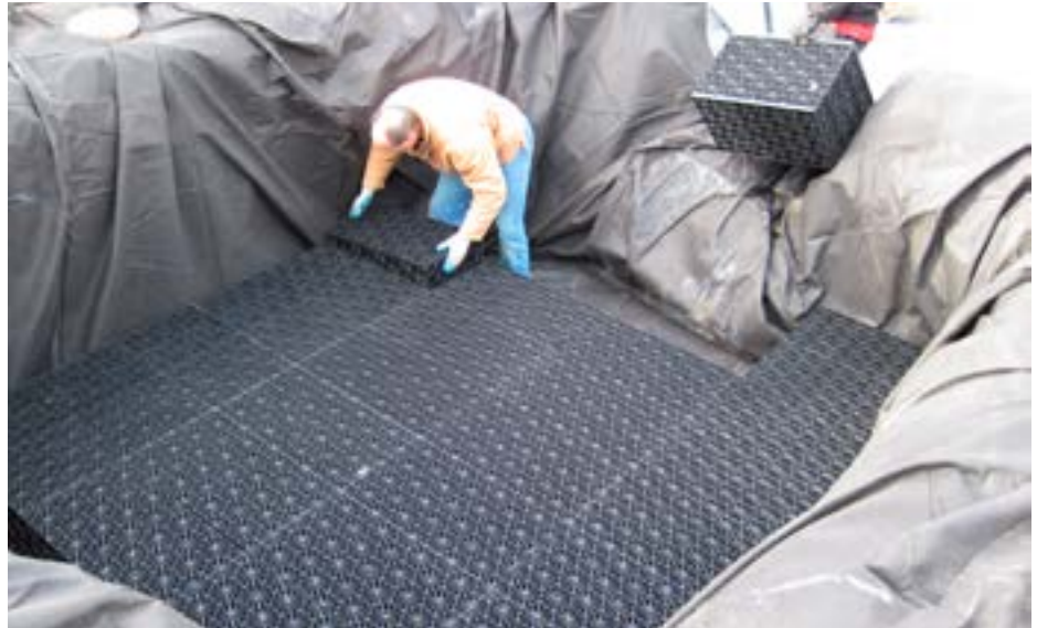
Figure 3. The pondless waterfall storage system makes use of EPDM pond liner and protective geotextile underlayment, with Aquablox providing structural support for the pond so it can be buried under gravel. PHOTO COURTESY OF LAKE WASHINGTON INSTITUTE OF TECHNOLOGY
