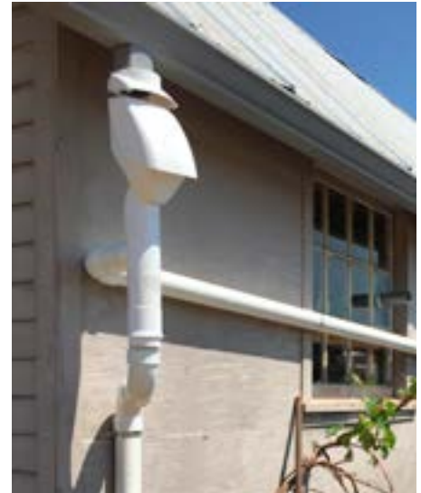
Figure 2. Seamless gutter with first-flush downspout diverter allowed the first several gallons of each rainfall event following an extended dry period to bypass the storage basin. The first flush of rainwater carried the majority of the particulate accumulated on the roof in the previous dry spell, and sent it to the storm drain as the same as a standard gutter. The diverter sealed off automatically after the first flush and started re-directing the rainwater to the cistern.
